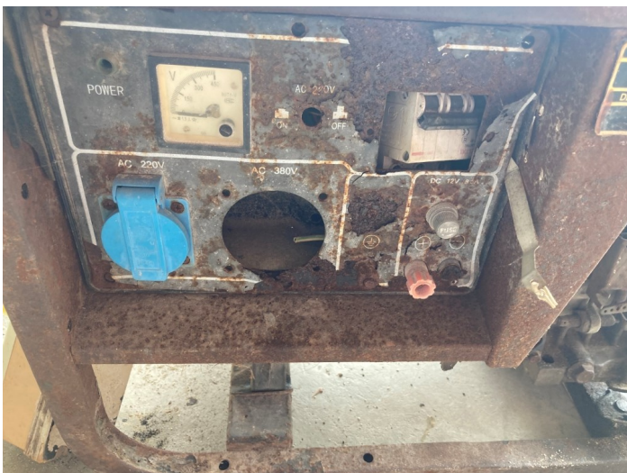
T32EU Emergency Backup Generator
